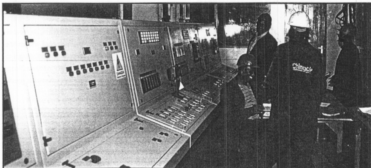
Diffuser control room
