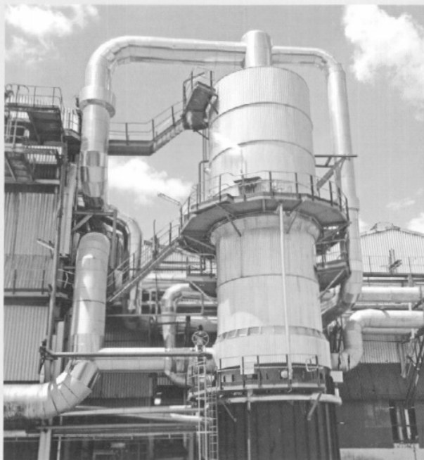
The new Evaporator for sugar extraction.
