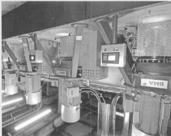
The newly installed Centrifugal Station
