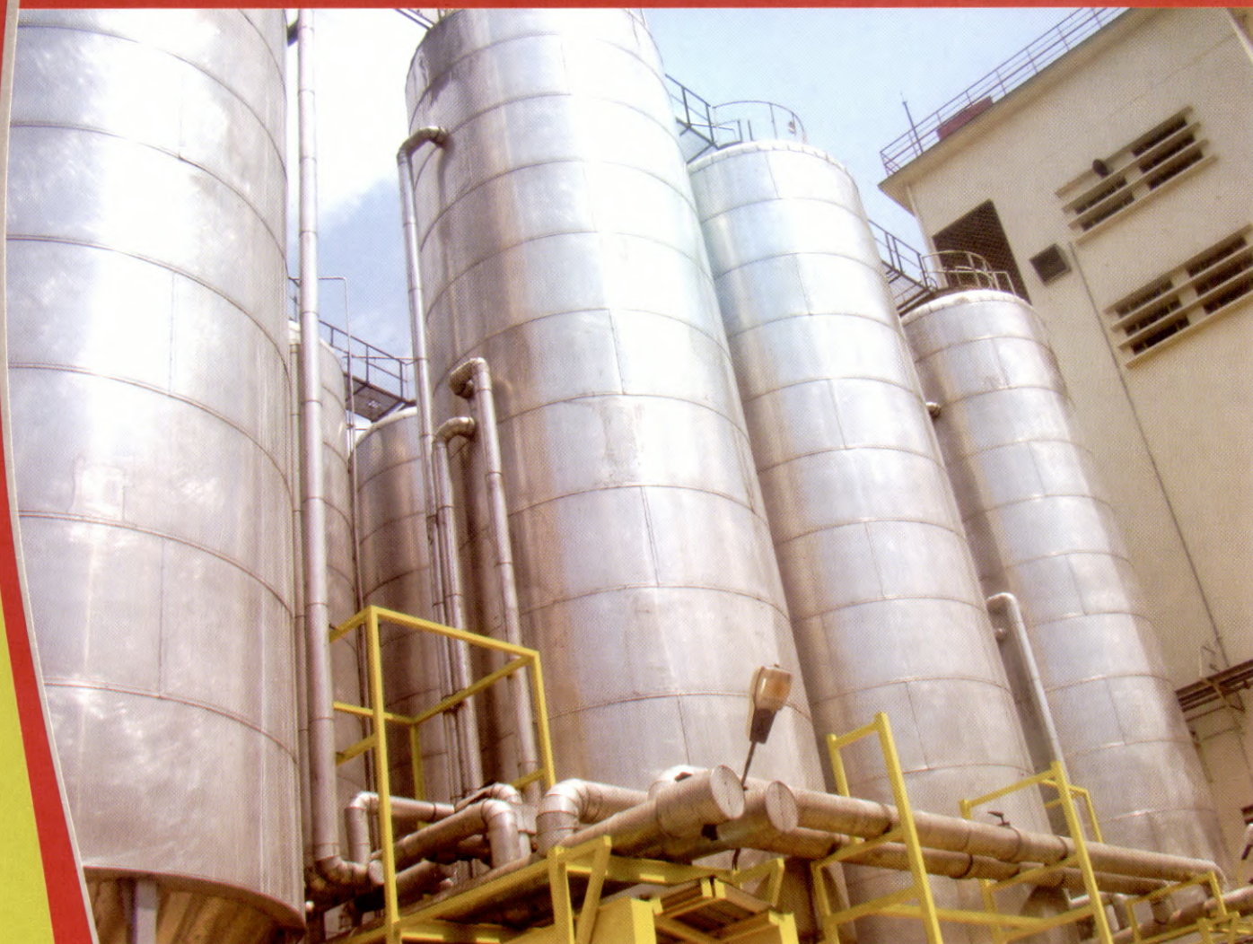
Dual Purpose Vessels at the Uganda plant
