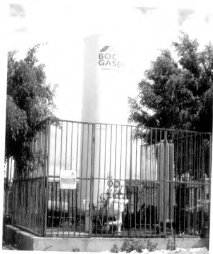
Installations on customer sites save costs for the customers and bring about service delivery efficiencies.
