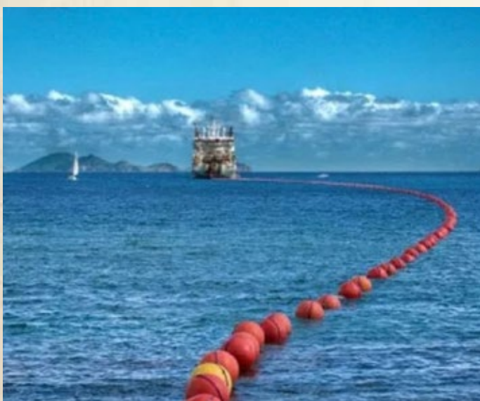
IPS Cable Systems Limited (Seacom)
