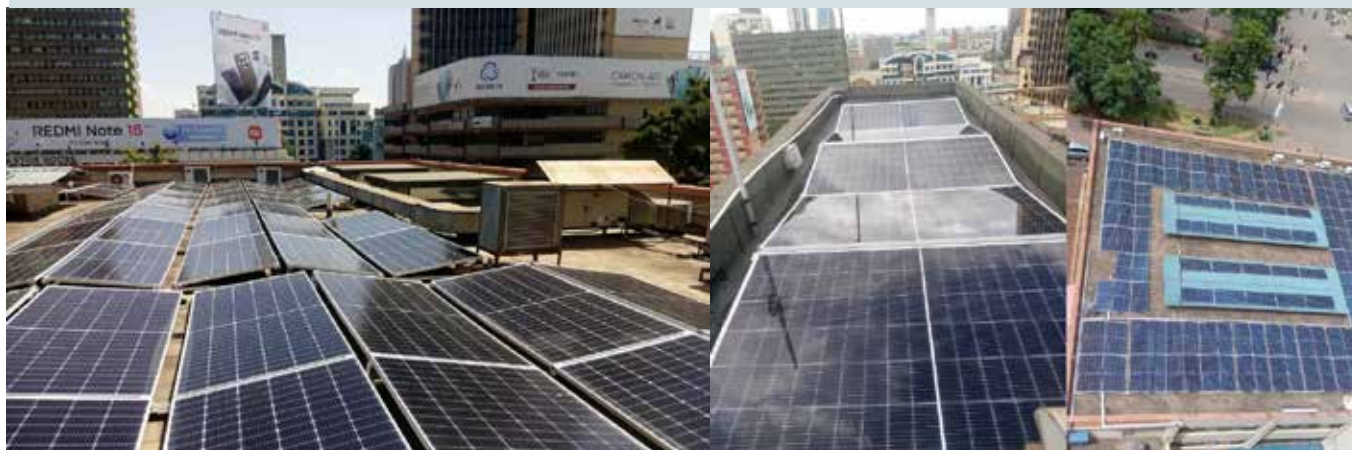
A snapshot of the solar panels installed on various sections of the roof of our Head Office at Rehani House.
