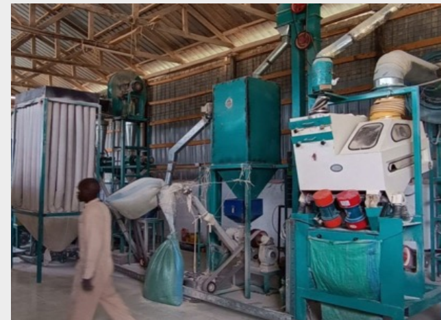
A 28-tonne maize milling machine installed at Tamkal
